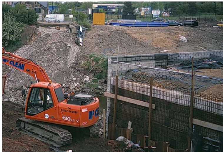
Fig 2: Temporary steel mesh panel wall erected to allow the demolition and removal of the existing structure
