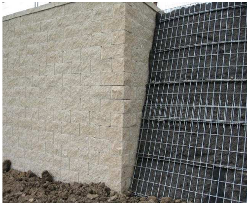
The black geosynthetic face liner retains the topsoil veneer prior to the vegetation getting established.
